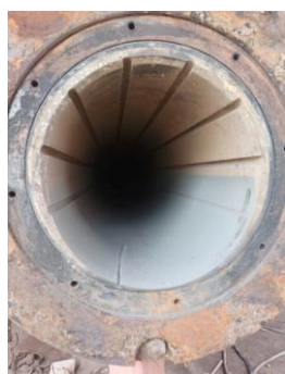
Figure 5. Vessel 8 (Viet Thuan, Tra Vinh river) after 2 years: Severe three-body abrasive grooving across all three bearing stave sections caused by sand ingress from unfiltered cooling water (TSS 380-520
