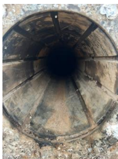
Figure 1. Vessel No. 1 (VTB Giang Hai) after 3 years operation: bearing surface - uniform shallow wear; AISI 316 shaft sleeve - slight scratches on the surface
