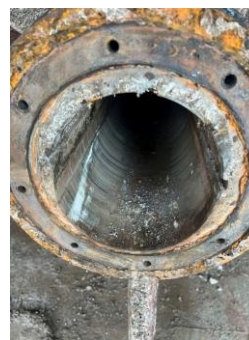
Figure 3. Vessel 6 (Hoang Gia tugboat) after 3 years: bearing bore with deep circumferential scoring from dry-running; AISI 316 sleeve with severe abrasive grooves and corrosion pits
